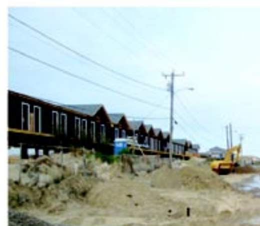
Photo 4. Back-filled water line trench in front of WHYC cabana construction, awaiting additional excavation for other utilities.
