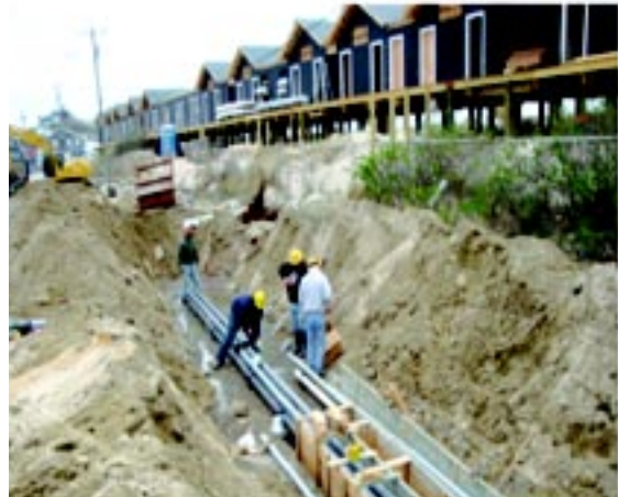
Photo 3. Placing conduits and forming for concrete to be poured around the conduits. This results in a protective “duct bank.”
