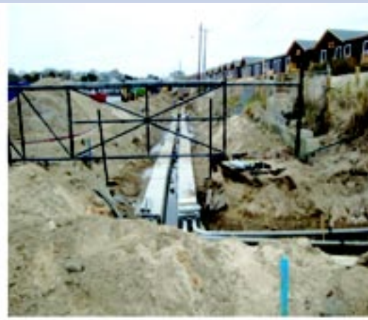
Photo 2. Looking down Fort Road from the Misquamicut Club Beach Club gate toward Larkin Square. Concrete-encased conduits in trench.
