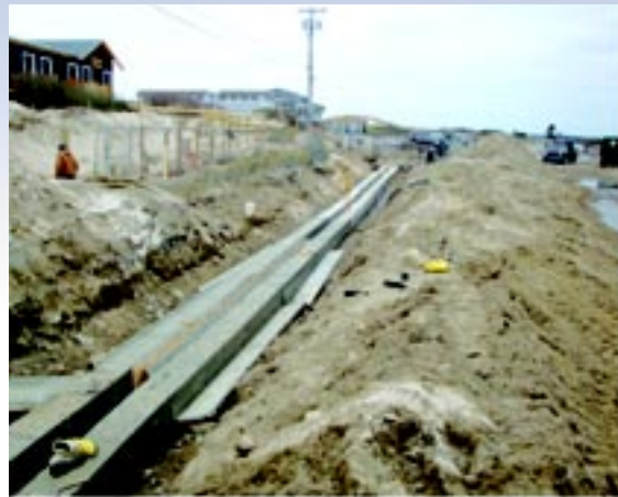
Photo 1. Looking out Fort Road toward the Misquamicut Club Beach Club. Concrete-encased conduits in trench, ready to be back-filled.
